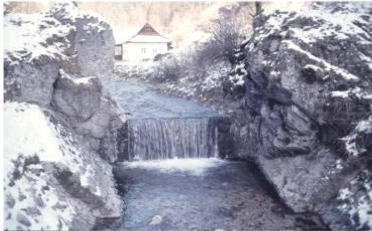
Fig.3 Weir carved in the rock in the torrent control Jelenec
